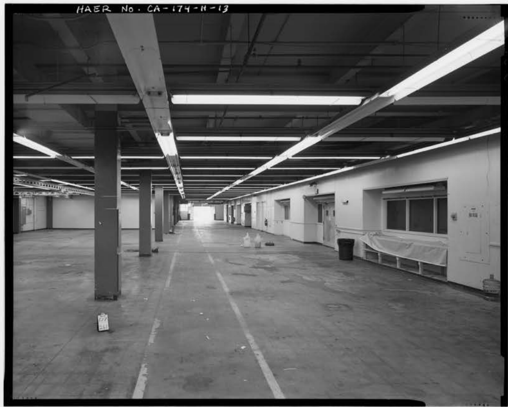
Large room with two-axis fluorescent lights in the Hughes Aircraft Company radar building, Los Angeles, California. Photograph by David De Vries, 1995. (Library of Congress, Prints and Photographs Division, Historic American Buildings Survey)
